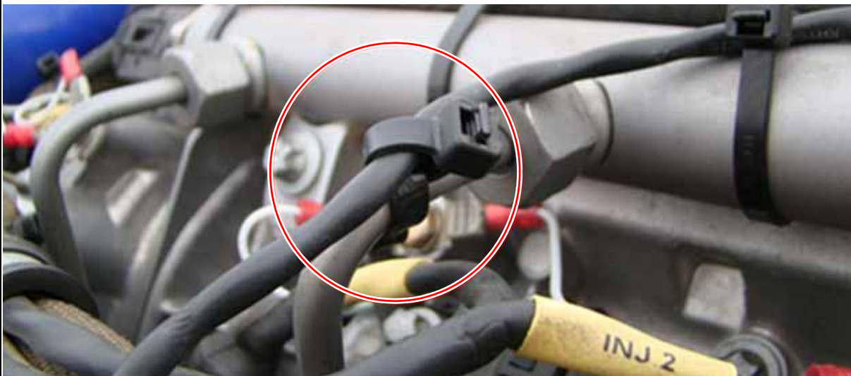
Figure 3 non-approved attachment: rail pressure pipe
