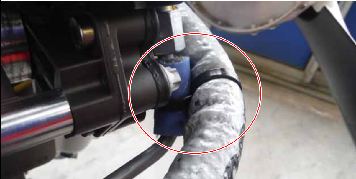
Figure 6 non-approved attachment: rail pressure pipe hpp to rail
