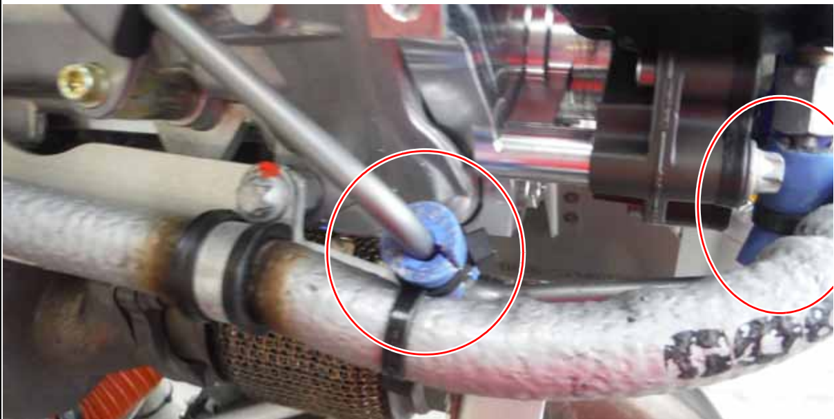
Figure 5 non-approved attachment: rail pressure pipe hpp to rail
